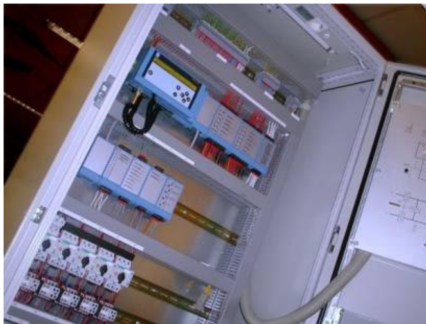
Illustration 1: Modern control computers with fully integrated Internet technology are being introduced into building management systems
